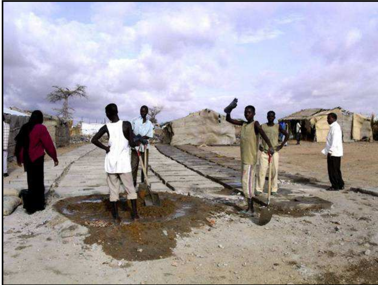
IDP youth construct latrine slabs in Kass, Sudan, as part of an OFDA-funded livelihoods program (Photo by Laura Chapman, USAID).
